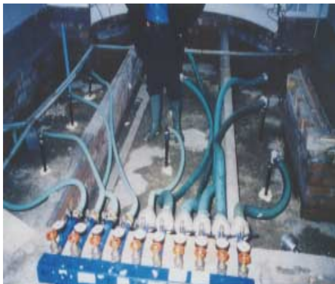
Photograph 2: remediation in action inside a property showing boreholes connected to vacuum extraction system (floor boards and joist removed) (G Madden)
