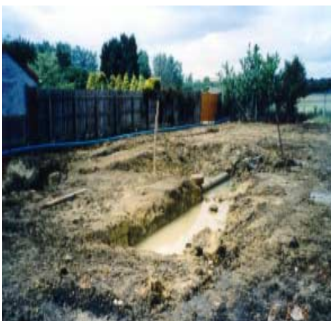
Photograph 1: fuel supply pipe line exposed (G Madden)
