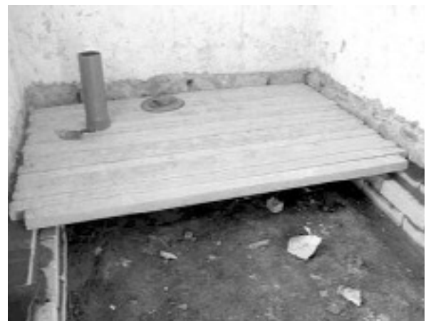
Room used as a 'radon sump', showing concrete lintels installed across the width of the room to create a false floor
