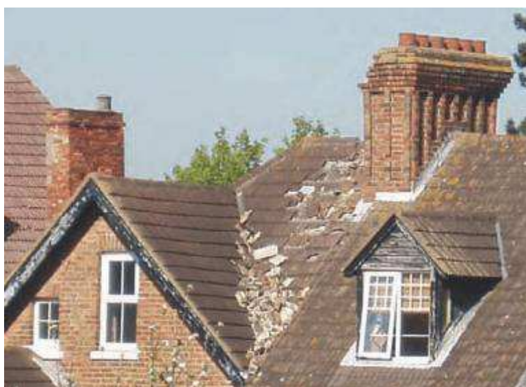
Figure 1: Chimney and roof damage in Folkestone (S Sargeant © NERC 2007)
